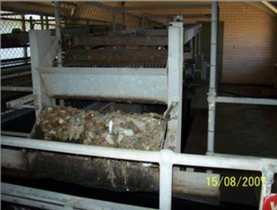
Inlet Screen, Sewage Treatment Plant, Bateau Bay, Australia.
