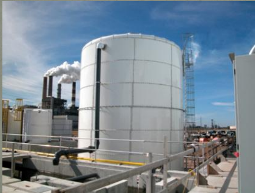
Tampa Bay desalination plant (power plant in background).
